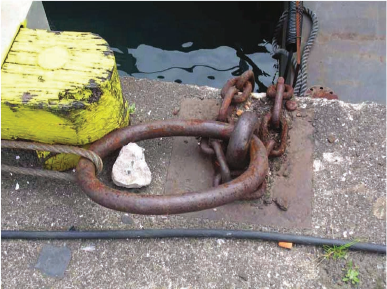
Eye-pin and ring fitting and toe rail (painted, left), North Wharf.
