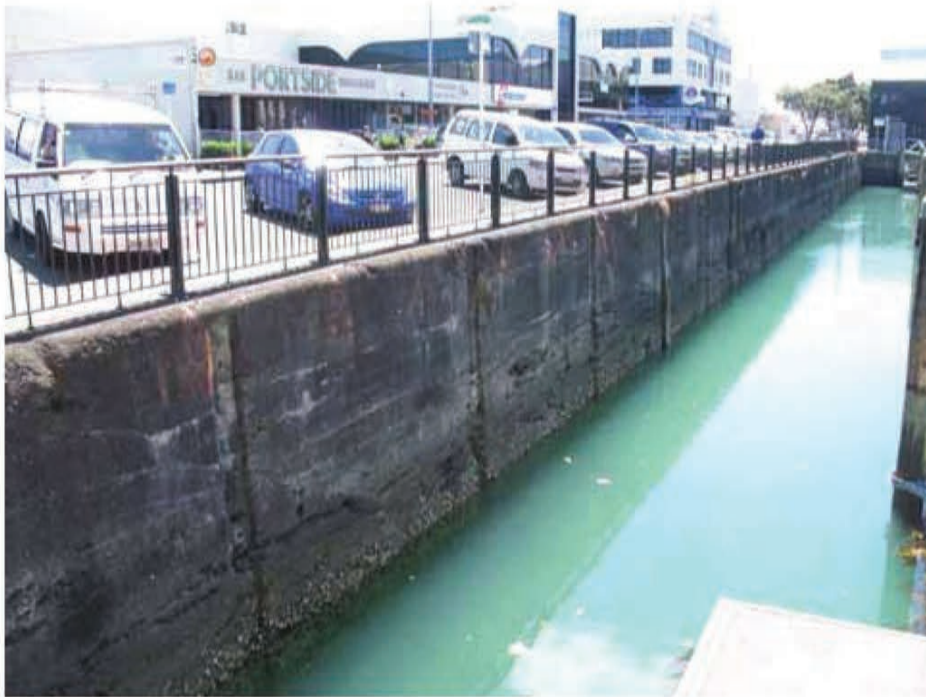
Intact section of Julian's wall, topped with modern balustrade. Note recesses for fender piles and ladders.
