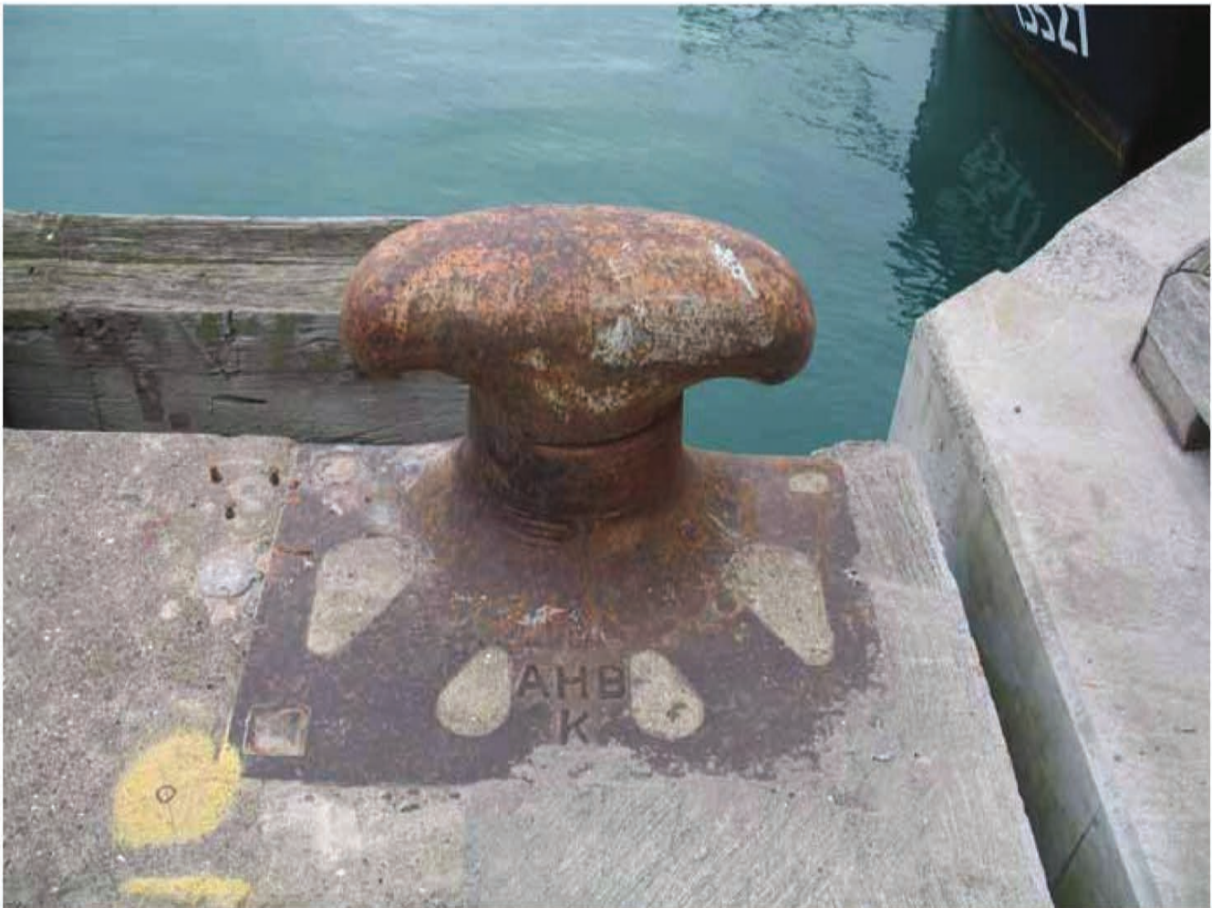
Type K bollard at eastern end of North wharf. Note textural difference between exposed aggregate surface of the historic wharf (far left) and modern wharf to right.
