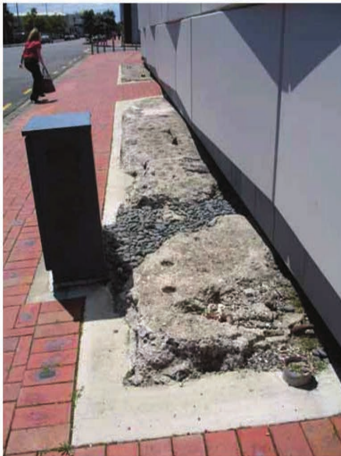
Sections of the top of Julian's wall that have been retained during construction of modern footpath between Viaduct Harbour Ave and Fanshawe Street.
