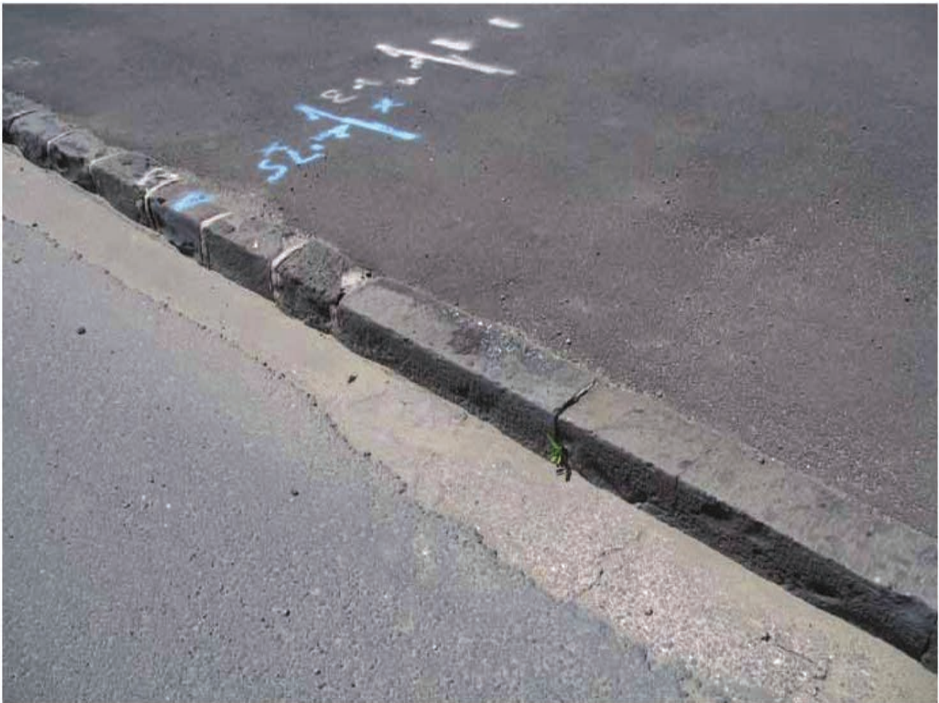
Bluestone kerbing , Beaumont St: Kerbing with original stones & detail on right, modern replacement on left.
