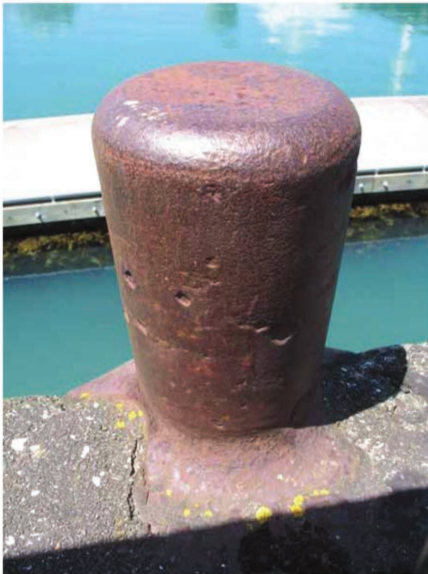
One of two remaining bollards on the exposed section of Julian's wall.
